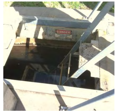
Figure 37 In-ground clear water tank
