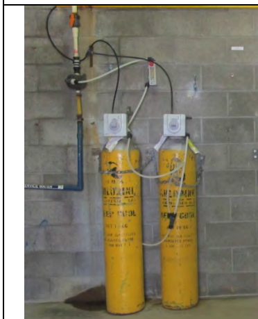
Figure 38 Chlorine gas cylinders
